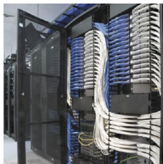
Figure 1. Production Data Center
