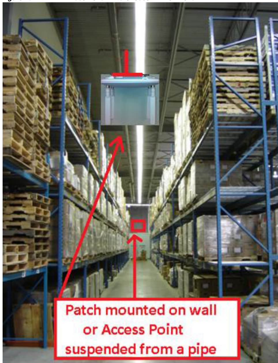
Figure 28 AP Placement in Warehouse Environment
