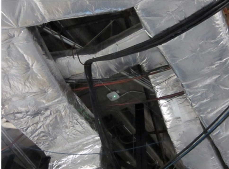
Figure 79 Example of a poor installation – Access Point is too high & buried in conductive foil
