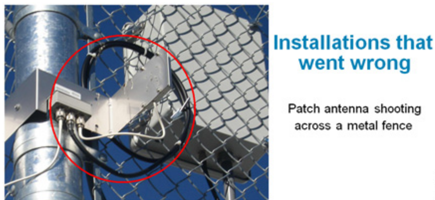
Figure 76 Patch antenna against a metal fence
