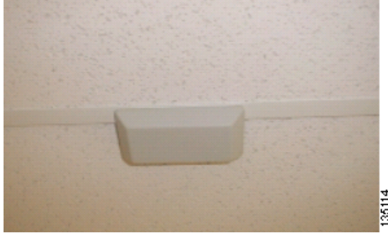
Figure 5-6 Patch Antenna Mounted on a Suspended Ceiling
