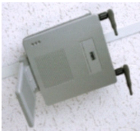
Figure 5-3 Access Point Installed on a Suspended Ceiling
