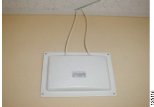
Figure 5-4 Patch Antenna Mounted on a Wall
